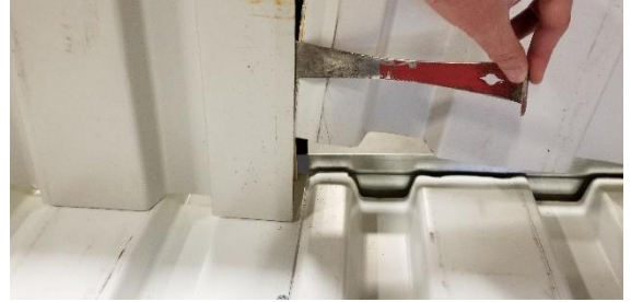
Figure 14: Trim Pry Bar used to help start inserting the tenon side into the channel side of the previous panel
