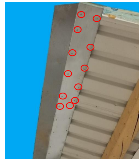
Figure 55: One side of roof with Ridge support angle installed underneath while panels are supported on a temporary wall.
