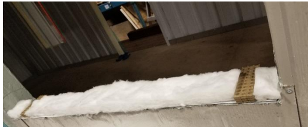
Figure 76: Fibreglass batt insulation on the sill cut to fit around the shims
