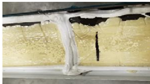
Figure 49B: Air barrier at the eave end, down the side and across the lower lip of the roof panel. A mono slope roof will require this bead above the wall at the high end in the same manner
