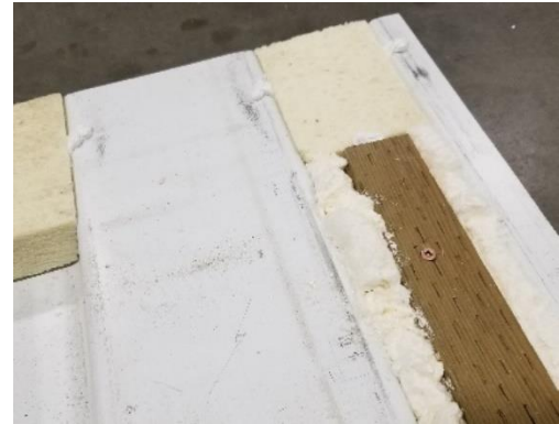
Figure 52: Structural lumber installed in flute above wall sealed with sealant and fastened with deck screws.
